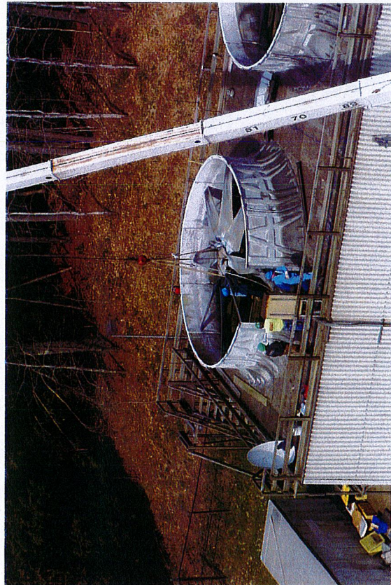
Bottom left photo of the old ash metal recovery magnets the new magnet (orange) is a permanent magnet and stronger than the old magnet on the left. Bottom left photo of the cooling tower repairs that took place during the shutdown. The fans and motors were removed and parts of the wooden structure were replaced.
