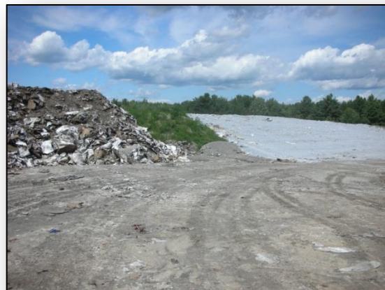
On the left is a pile of wetlap; on the right is the existing MSW storage berm covered with shredded wetlap.
