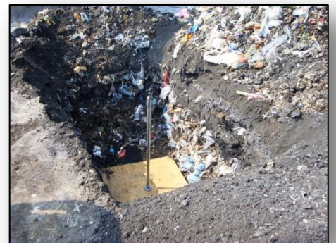
A new geological monitor is placed in a pit to measure ground movement. Continued on next page...
