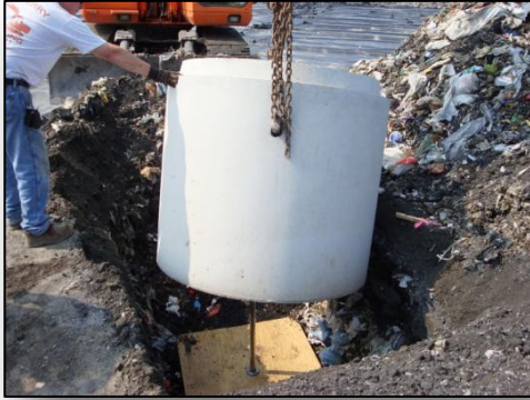
In the next step, a large concrete protective cylinder is placed around the measurement device...
